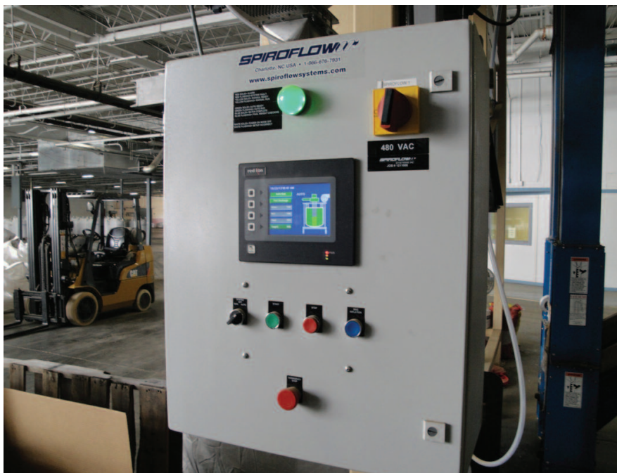
Each bulk bag filler has a control panel with digital weighbatch controls, a slide-gate valve position control, and a bag inflation fan control.
