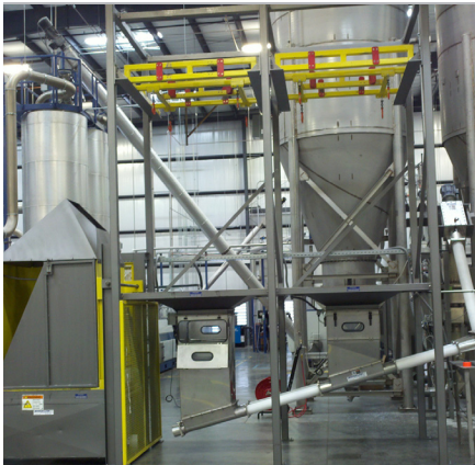
Box Dumper and two Bulk Bag Unloaders deliver flake material into mixing silos.
