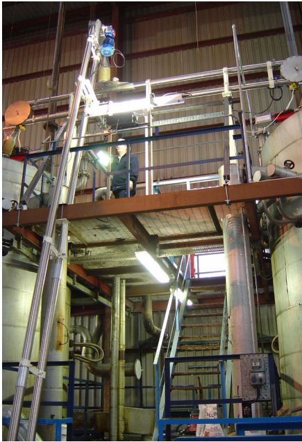
Typical Aero Mechanical conveyor installation with one unit transferring to another
