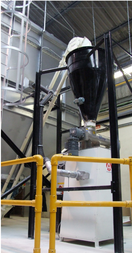
The Second Spiroflow Aero Mechanical Conveyor
