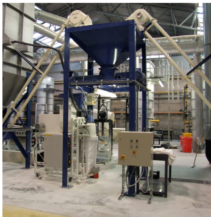
The Third & Fourth Spiroflow Aero Mechanical Conveyors
