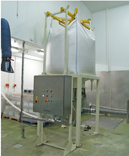
Bulk Bag Unloader with Flexible Screw Conveyor leading off through warehouse wall
