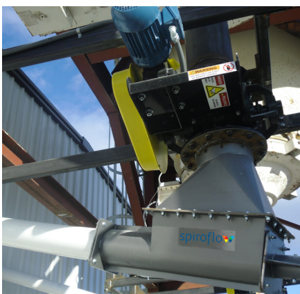
Spiroflow Flexible Screw Conveyors moves flour from silos.
