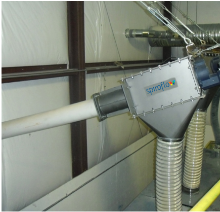
Spiroflow Conveyors installed through an exterior wall convey flour to a ribbon blender
