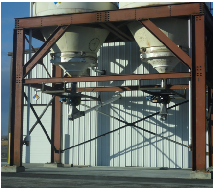
Twin Conveyors under outdoor silos.
