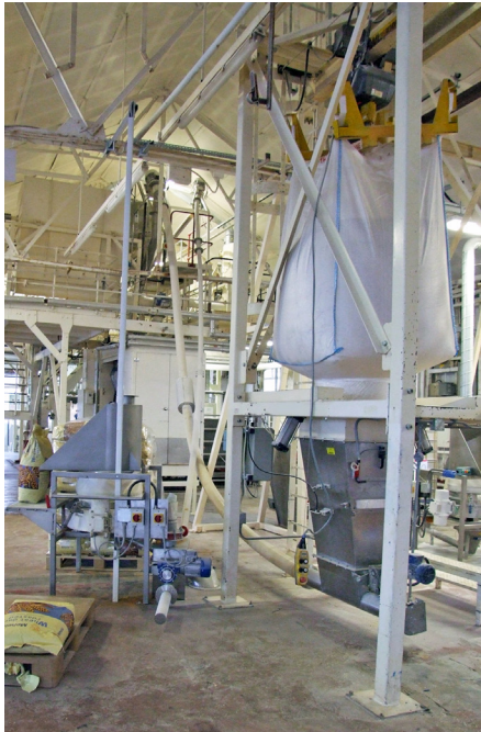
General view of the installation
