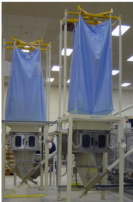
The two Bulk Bag Unloaders inside the Premier Foods factory.
