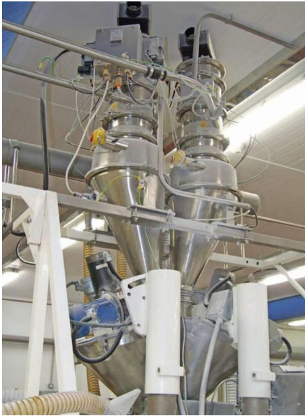
The vacuum transfer system to the packing machines
